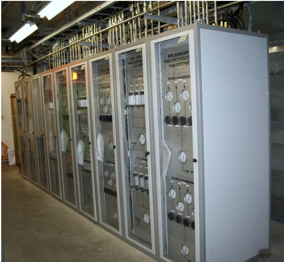
CMS RPC gas system in USC5
